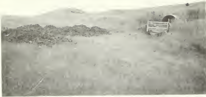
NORTH ENTRANCE, looking towards Southeast; Notice fill material cleaned out of pipe
